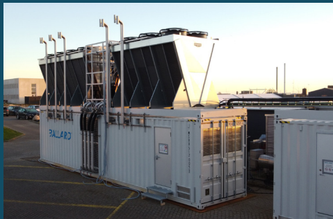
1MW decentralized power generation for EV charging
