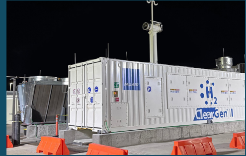
1.5MW back-up power at Microsoft data center
